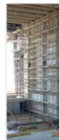
Casa Da Musica, Porto, Portugal, under construction 2002 TICO Structural Bearings and Bond Slip Sliding Bearings were specified.
